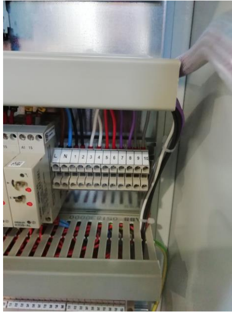
Terminal box condenser unit generator
