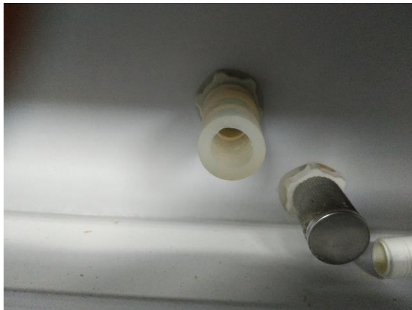
Pipe without the water collector
